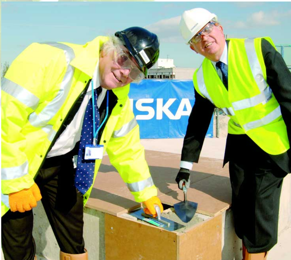
▲ Trust Chairman Brian Meakin (left) and Peter Coote, Executive Vice-President of Skanska UK, add the finishing touches to the roof of the DTC.
